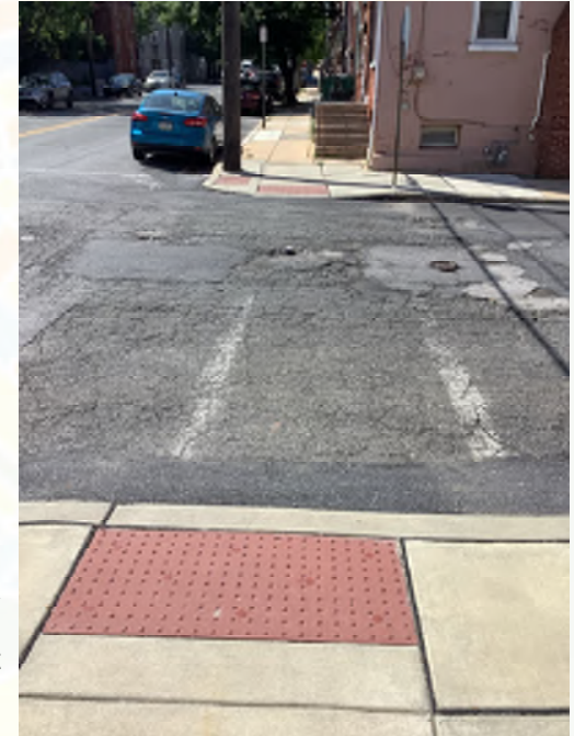
Curb ramps are in good condition, but crosswalk markings are broken and faded at Marshall Street and Fulton Street.
