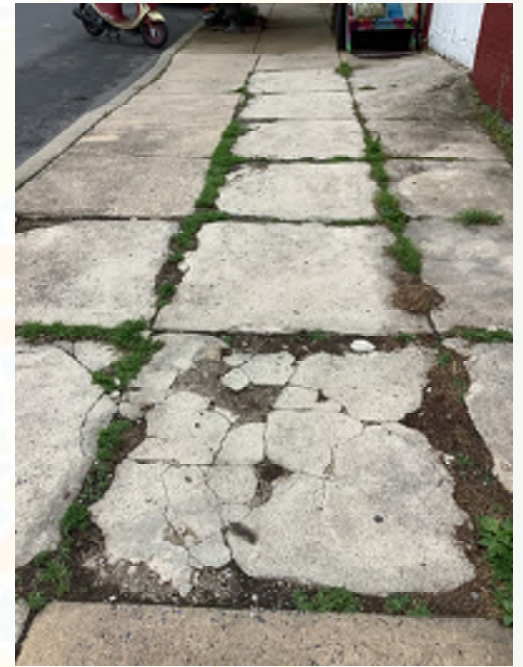
There are scattered sections of rough sidewalk, such as this one along Shippen Street near New Street.
