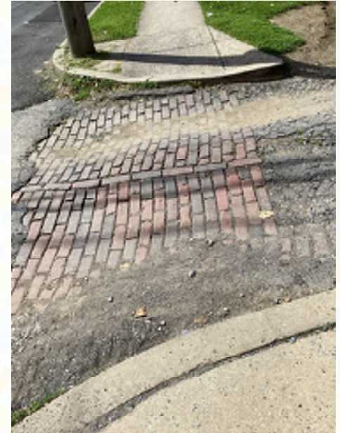
There are no curb ramps and the crossing surface is rough along Franklin Street near Madison Street.
