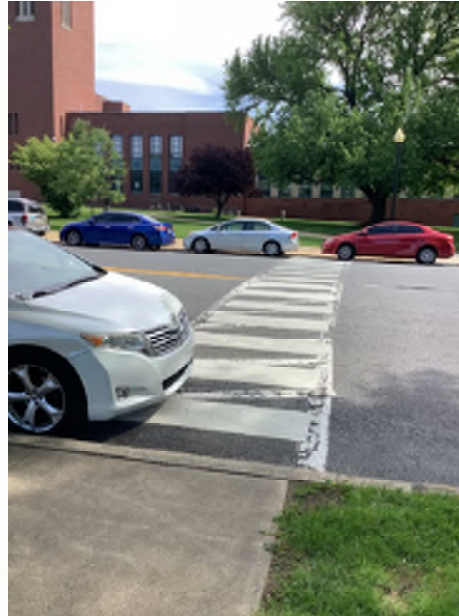
There are no curb ramps at several crosswalks along Reservoir Street near McCaskey High School.
