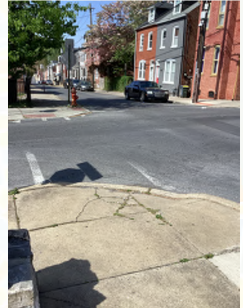
This curb ramp at Filbert Street and Vine Street is in poor condition and lacks the detectable warning surface (DWS) seen on the opposite side of the intersection.
